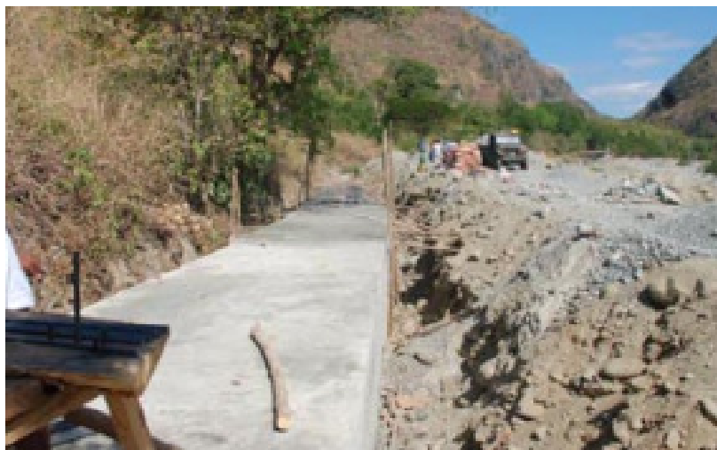
Shown above is the ongoing concreting of a DA-NIA funded tunnel type irrigation system in Abra.
