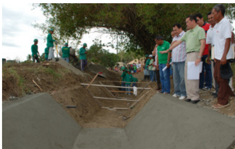
Agriculture Secretary Arthur C. Yap (2nd from right) inspects the construction of irrigation canals, at Bgy. Lataag, Laoag City, which forms part of the P8-million Laoag-Vintar River Irrigation System. Once completed in May, the project will irrigate 1,850 hectares and benefit 2,642 farmers.
